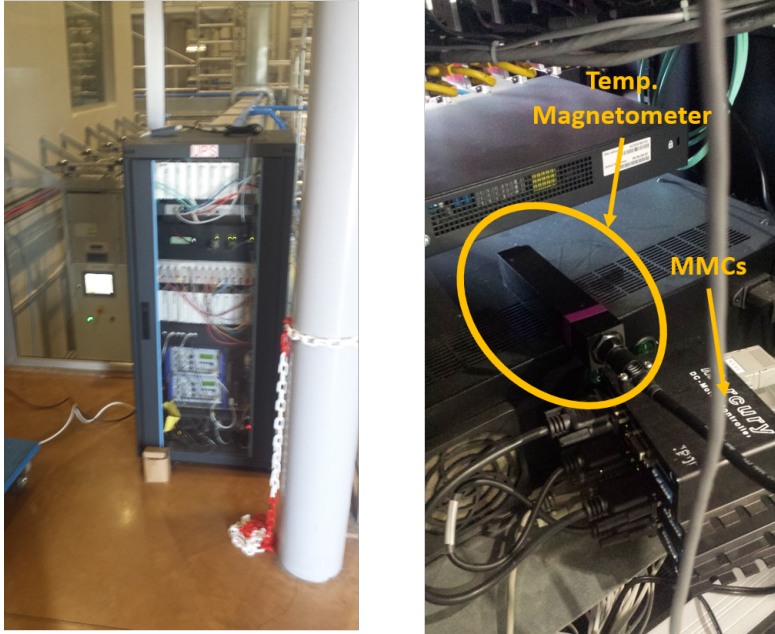
Figure 5: Left: Minirack Right: Mercury Motor Controllers and temporary magnetometer
