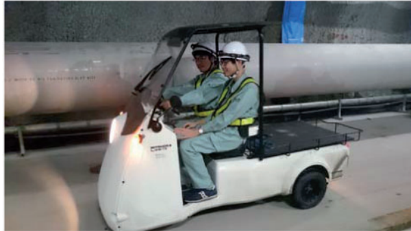
Fig. 10. Each worker is equipped with a helmet, work clothes, reflective vest, and headlight for work inside the tunnel. Small electric carts are used for the 3 km transport from the central area to the end station.
